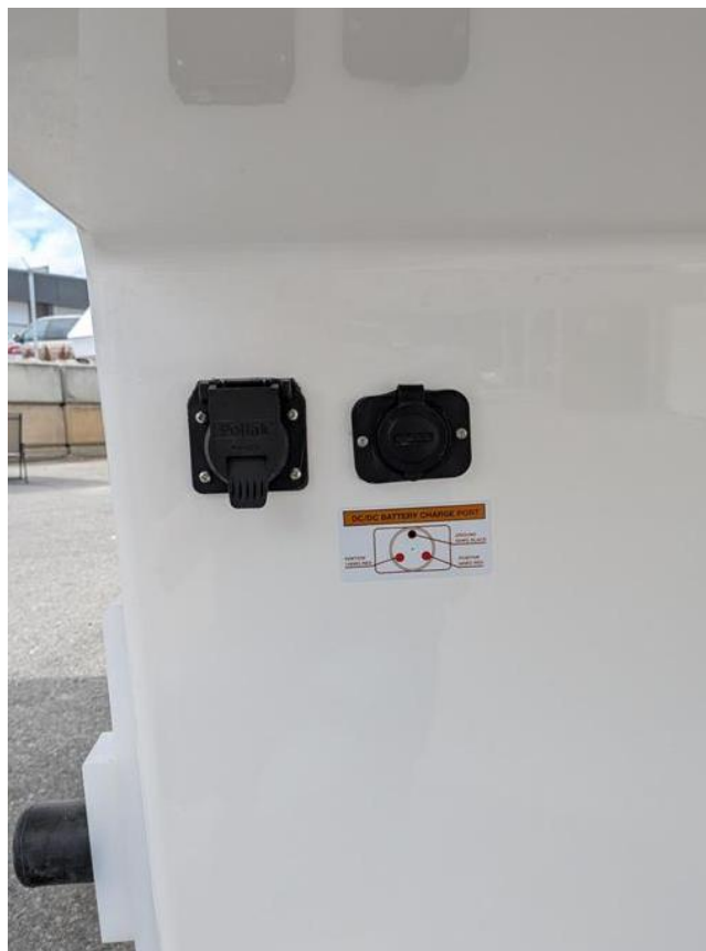
Figure 2, 7-Way Power Connection and DC-DC Charger Connection
