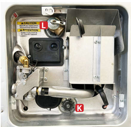
Fig#3 Water heater
