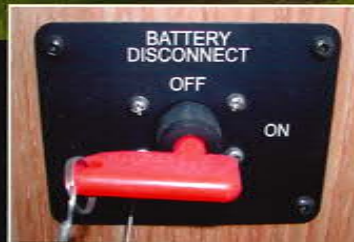
Battery disconnect switch.
