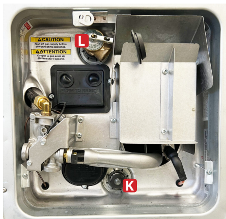
Fig#3 10-2 Water heater
