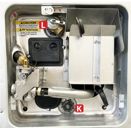
Fig#3 Water heater
