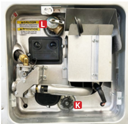
Fig#3 Water heater
