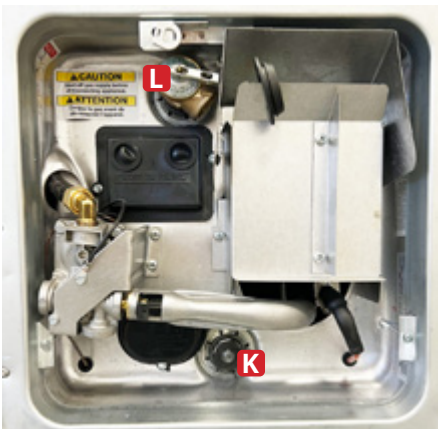
Fig#3 10-2 Water heater
